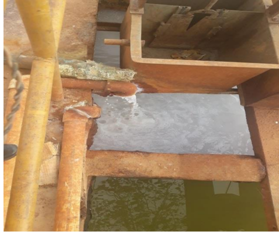
Segregated Lime & FeSO 4 Dosing in Physico-Chemical Treatment Section of CETP
