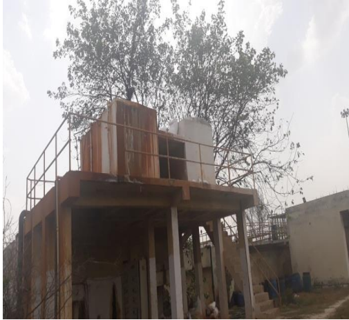
Lime milk & FeSO 4 preparation Tanks (Before)
